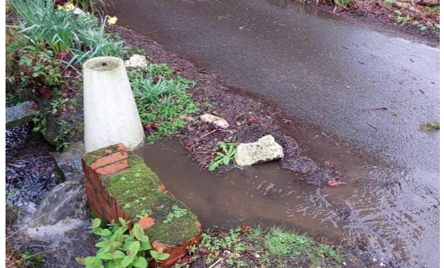
Figure 3 - Water flowing off Water Lane into ditch, under the road and across to ditching on Preston Farm 2 nd March 2024
